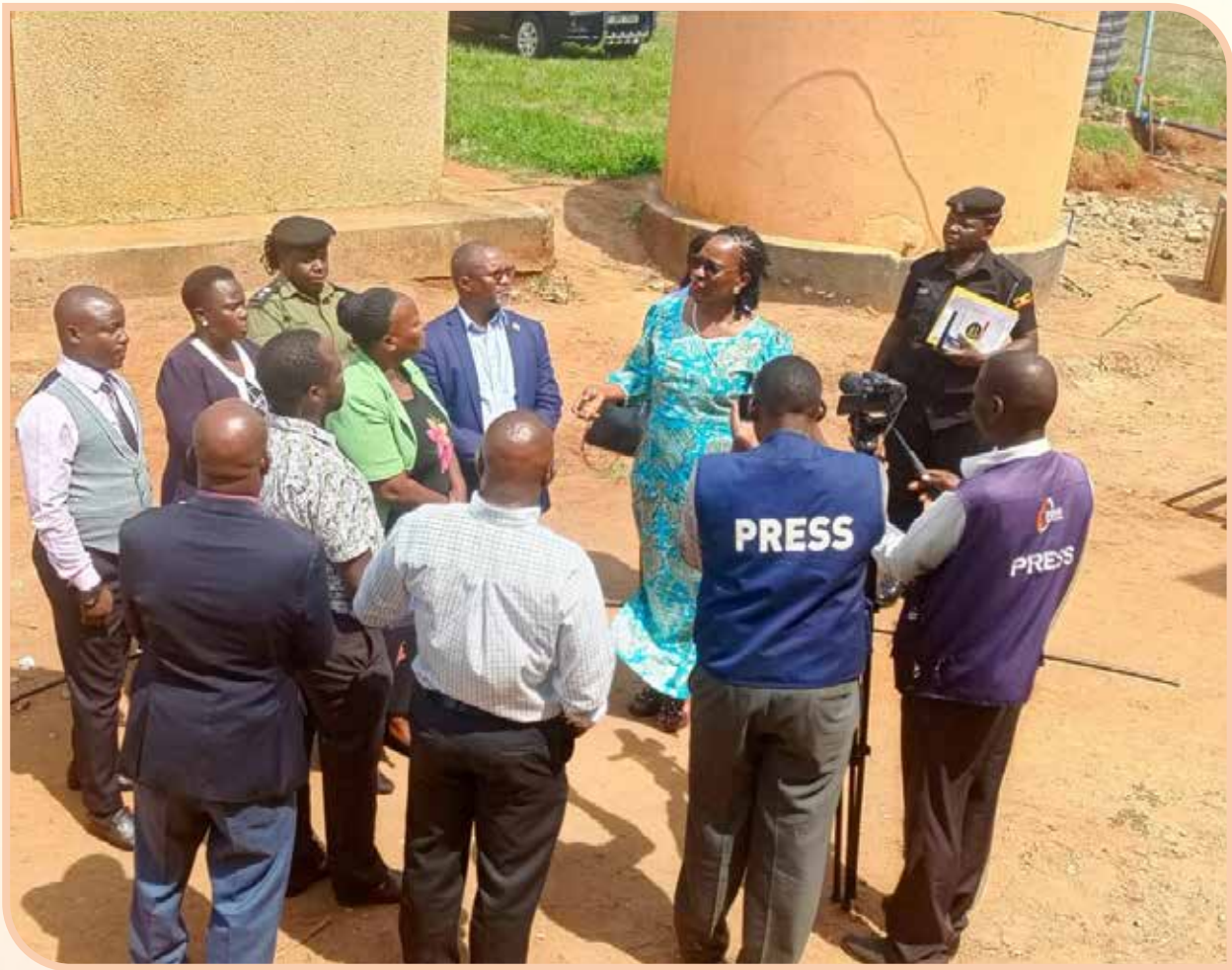
Deputy IGG Mrs. Anne Twinomugisha Muhairwe addresses Journalist during inspection of construction works at Kalungu District Local Government Headquarters.
